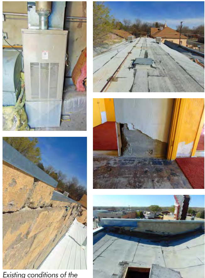
Existing conditions of the roof and building interior.
