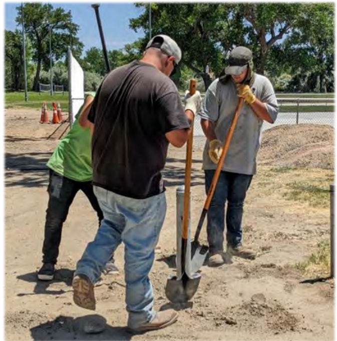
Alternate 1. Post and cabling at parking area.
